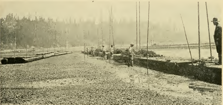
Hand Leveling.—Scows were loaded by cutting down high part of bed to desired level, then floated to part to be filled and shoveled off.
